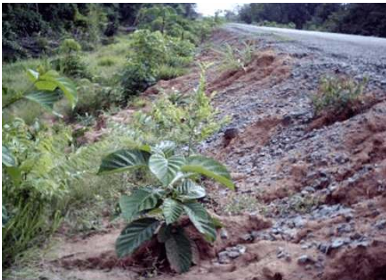
Fig. 2: Access road to a flowstation in the study area. Notice the 2-4m road embankment.
