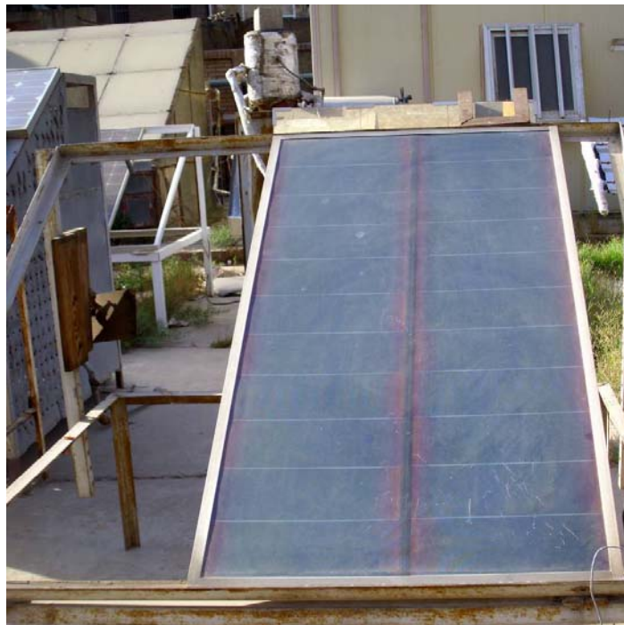
Fig. 17: Photograph of PV module 1.
