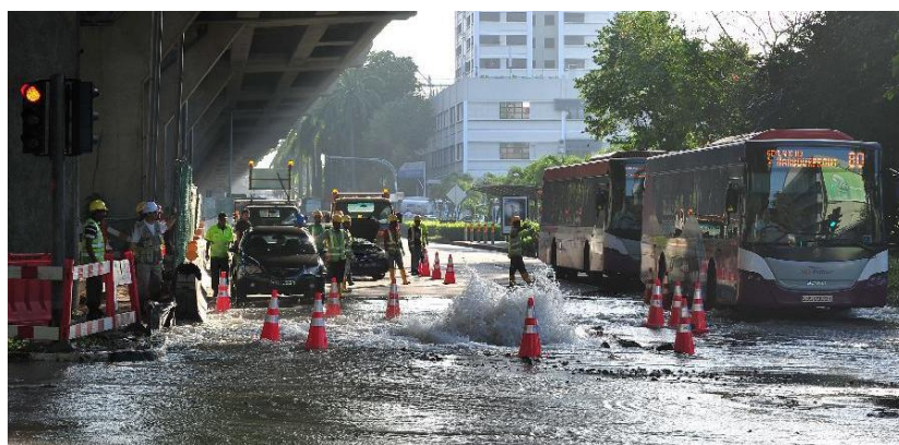
Fig. 4: Poor road built on the middle of the road.
